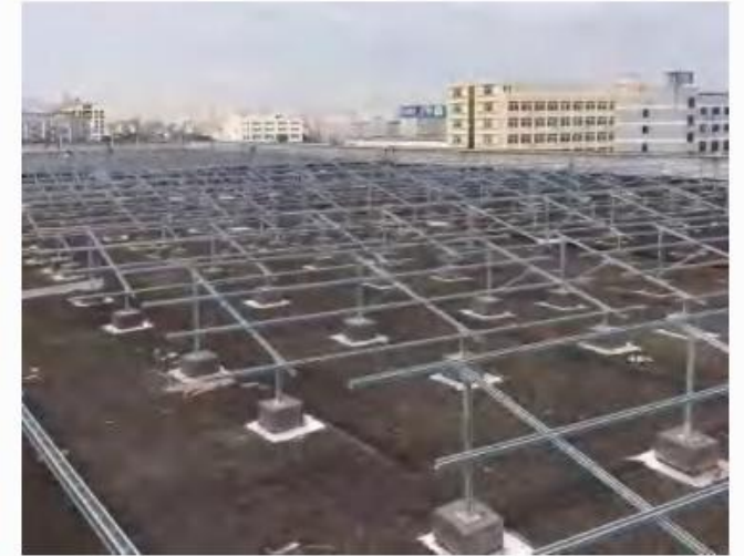
3.2MWp Flat rooftop
