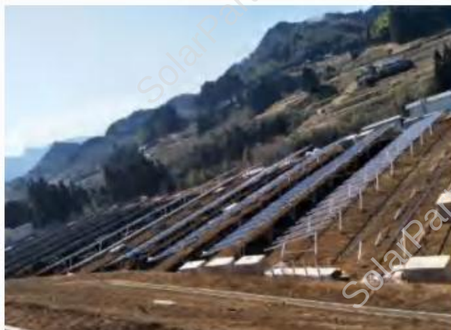
2.3 Mwp in Japan
