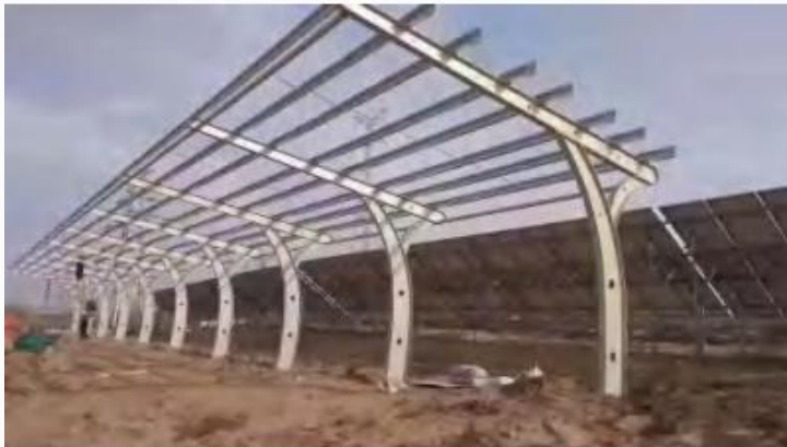
800KW FUJIAN, China
