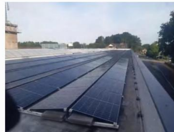
800kw in Mauritius
