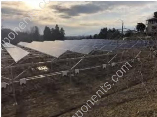
500KWp solar Farm Japan
