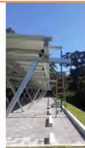
195kw Solar Caport in Italy
